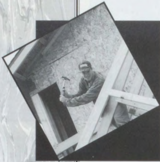
Learning construction techniques, Jesse Huffman is setting trusses on the house during his building trades class.
