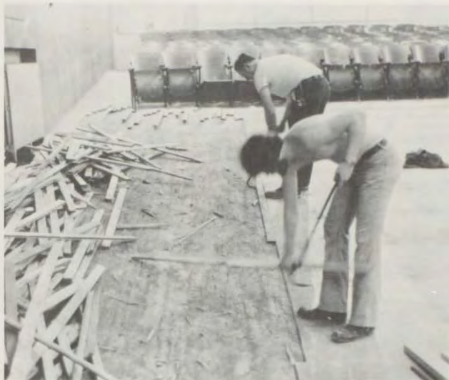
Rick and Ferd Kleeman help remodel the auditorium by tearing up floorboards.
