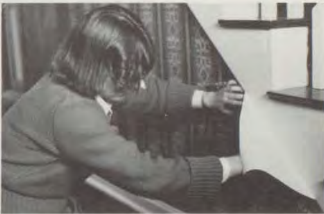
Becky Claise puts the finishing touches on a tight corner of this staircase.
