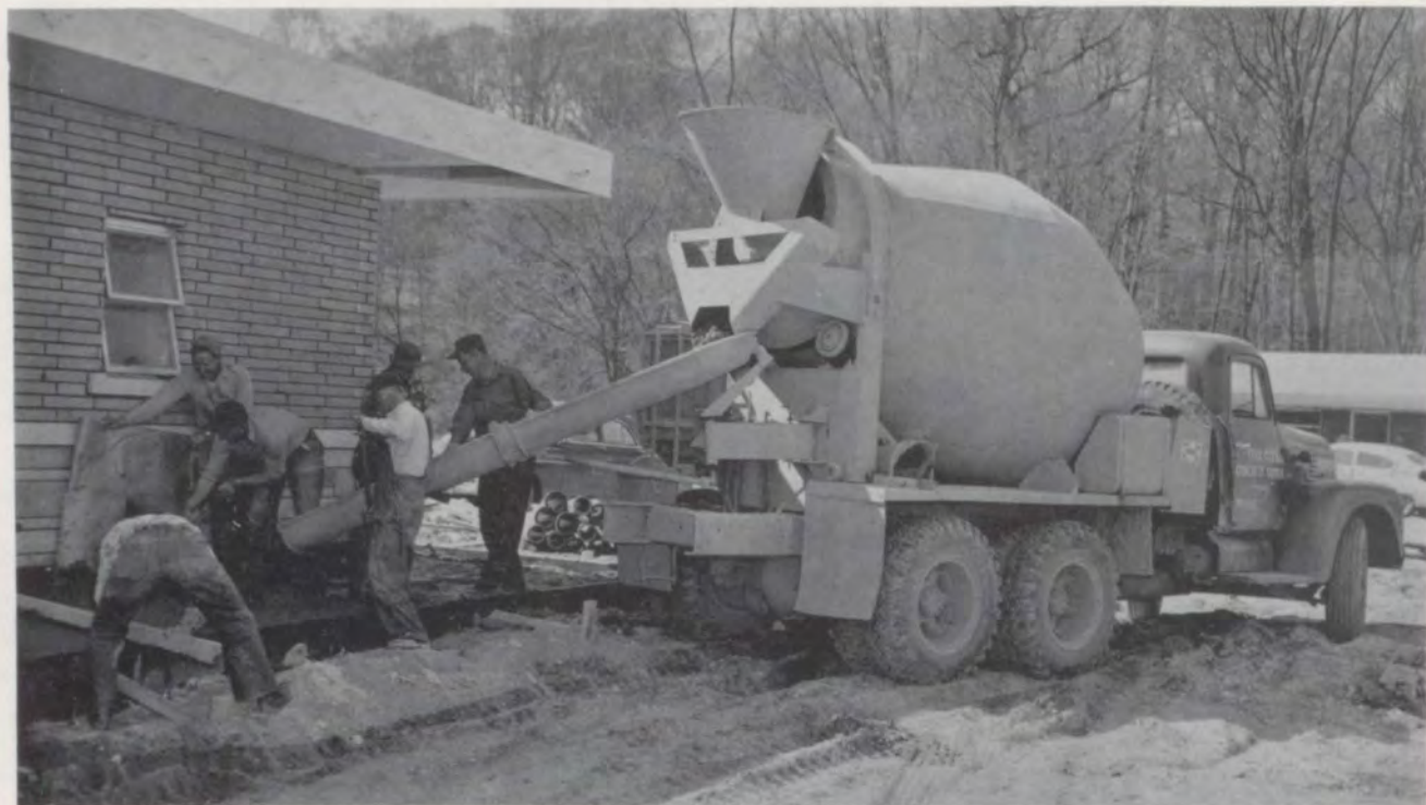
For ready mixed concrete in any amount or formula, at any time or place, call MULZER BROTHERS. Here, one of their big jobs is completing some walks at the new motel.
